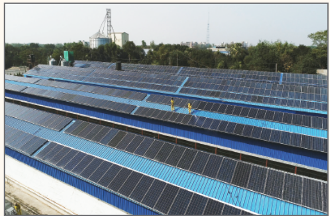
Rooftop Solar at Paragon Feed Ltd.
