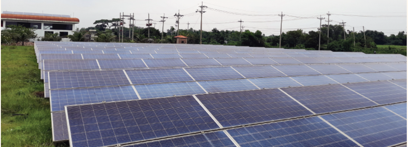
1.1 MW Rooftop Solar Project at Far East Spinning Mill, Madhabpur
